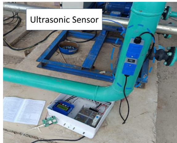
Figure 2. Ultrasonic sensor installation
